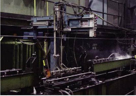
Squirter type ultrasonic inspection station on a weld-line at Wheatland Tube, Arkansas. MAC Echomac electronics are operating with this test system.
