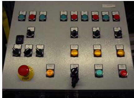
Conductor Control System
