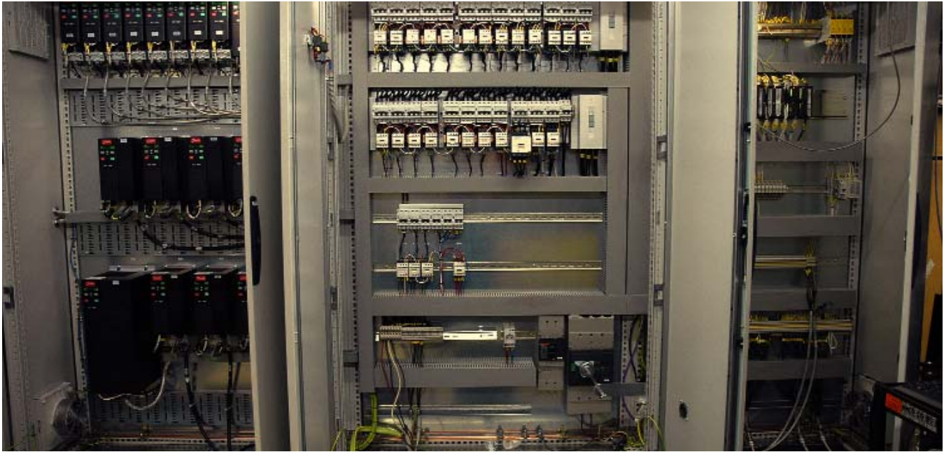
Conductor control system and PLC for the control of a MAC multi test system * Described on back cover
